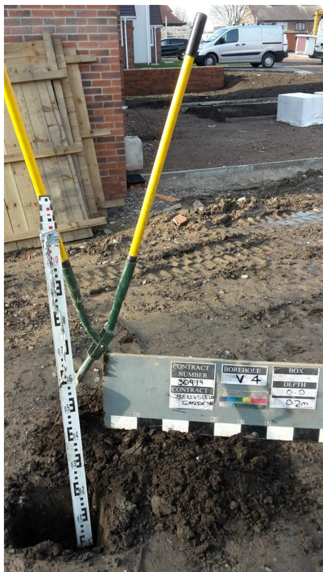
Photograph C: Location V4. Soil well in excess of 300mm
